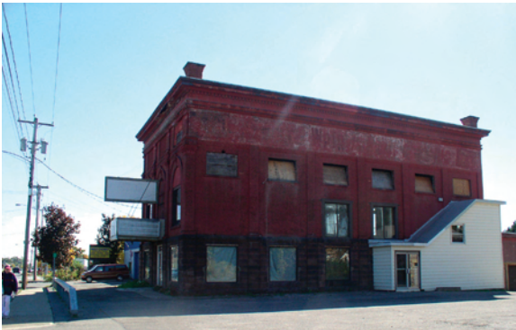
The oldest and arguably the most majestic building along the corridor has unfortunately fallen into a state of deep disrepair and neglect.
