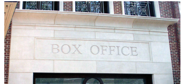
This sign in a traditional sign band location has recessed letters in cast stone, for a clean, quality look.
