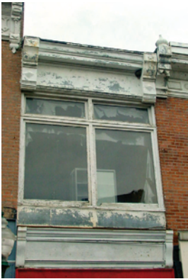
Building should be maintained in a good state of repair.
